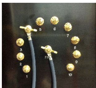
GPS360 Relay Connected to Rectifier AC
