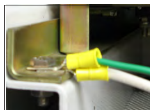
RM4015 Ground Connection to Rectifier Ground
