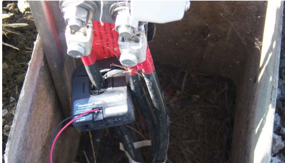
Figure A-2. Selectable Current Transducer - Installed
