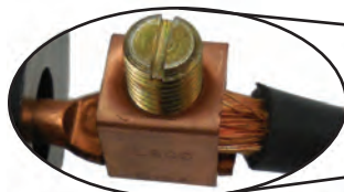
Welding Cables on Relay
