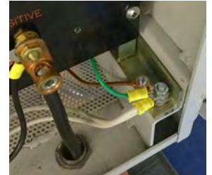
Common Ground Location on Rectifier Chassis
